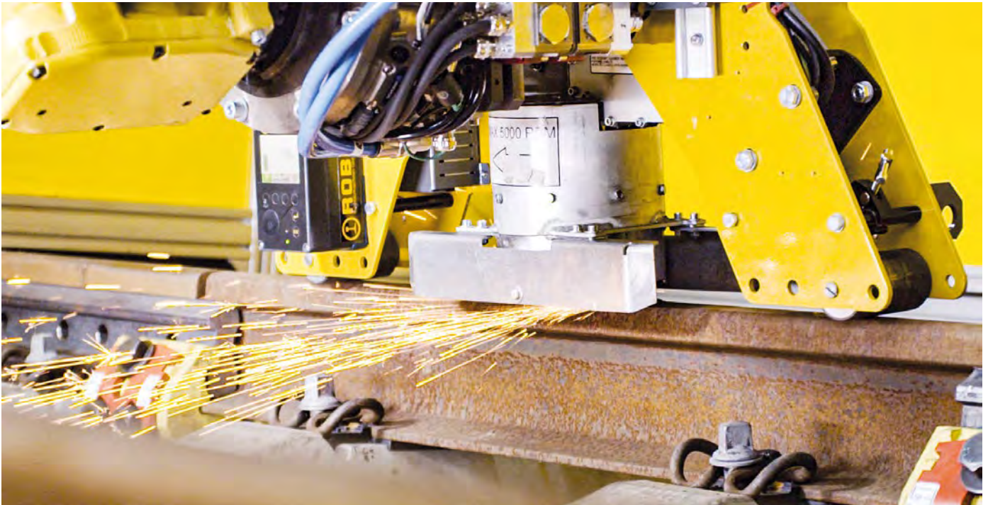
Fig. 6: Finish grinding of the facets on the surface of the rail generated during the milling process
