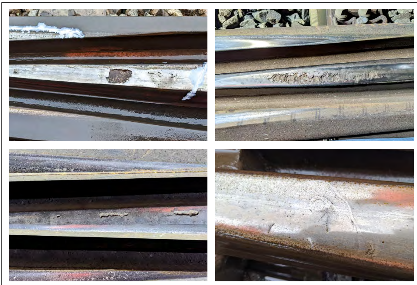
Fig. 4 (collage with 4 pictures): Turnout defects which can be remedied with automation: wear on wing rail and common crossing as well as breakage to the crossing vee on a previously repaired section | breakages to the vee crossing resulting from a wing rail that is too low/one-sided loading | cracks and breakages to wing rail and crossing vee | hydrogen-induced crack caused by incorrect preheating
